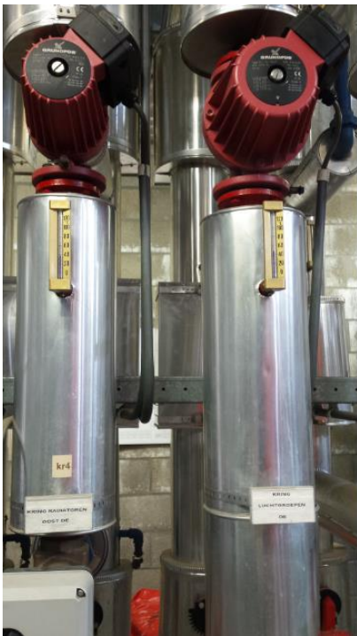
Figure 66: Part of the control system
