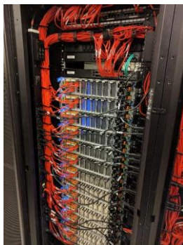
Figuur 22: Bekabeling Avamar backup servers
